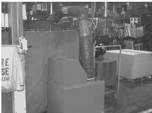
Figure 3. The portable exhaust ventilation unit. These units moved 740 cubic ft. of air per minute and were positioned to pull the fume out of the welder's breathing zone. The units are lightweight and are easily manipulated by employees. The combination of local exhaust and general ventilation reduced the amount of welding fume exposure by 51 percent. 28
